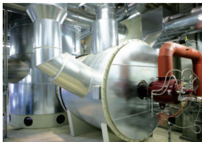
Vertical combustion chamber.
