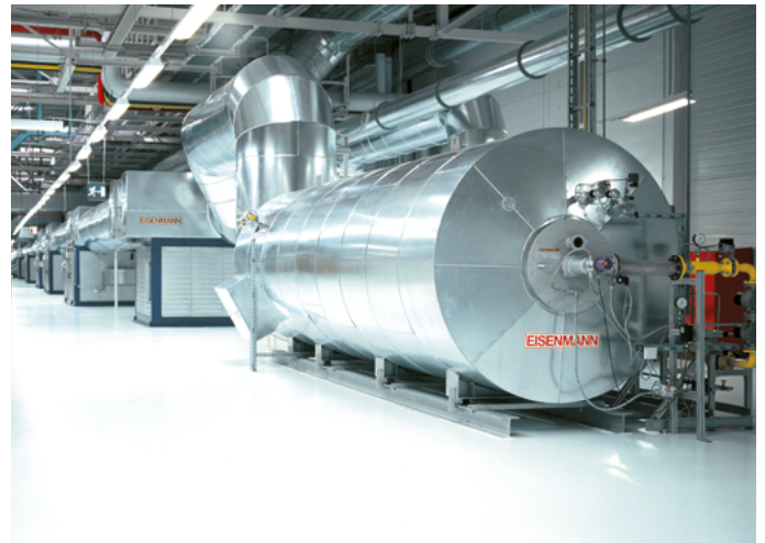
Thermal oxidation plant in the automotive industry
