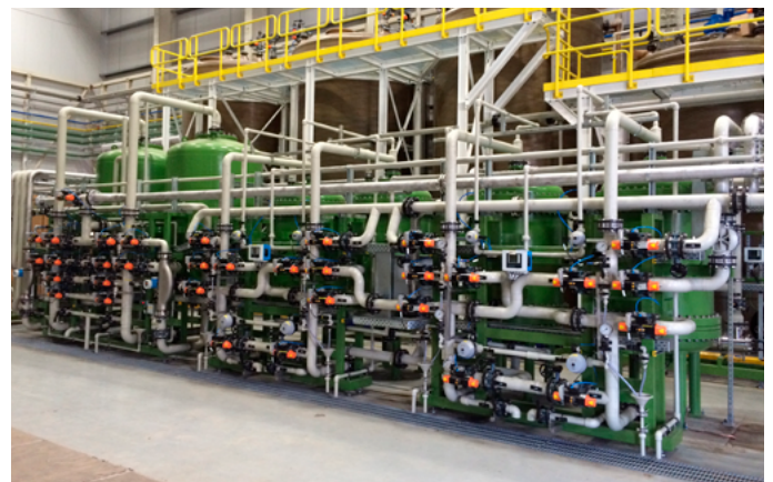
Rinse water recycling by ion exchange, capacity 25 m 3 /h.
