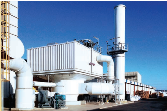
Regenerative thermal oxidation (RTO) with rotating distributor to minimize pressure fluctuations.
