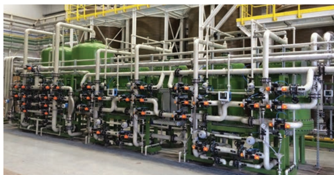
Rinse water recycling system with a capacity of 25 m 3 /h.
